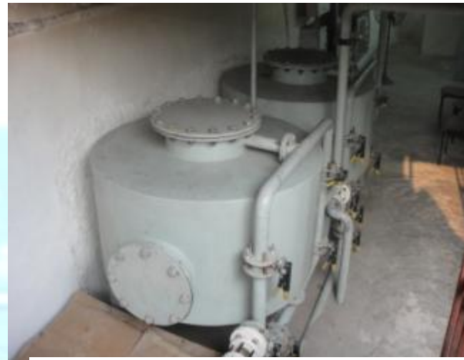
Activated Carbon Filters
