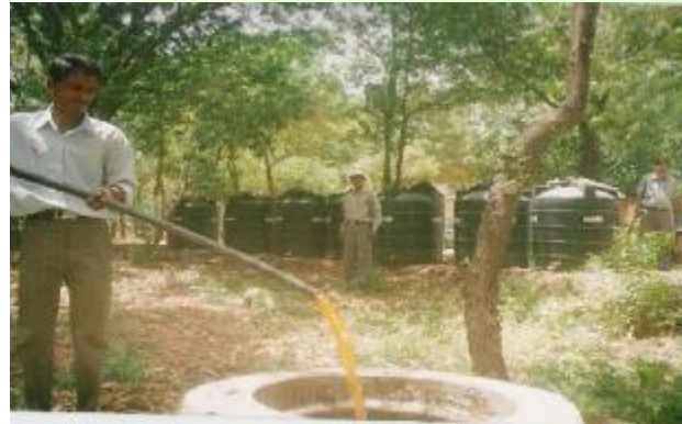
Bacteria dosing in the manhole
