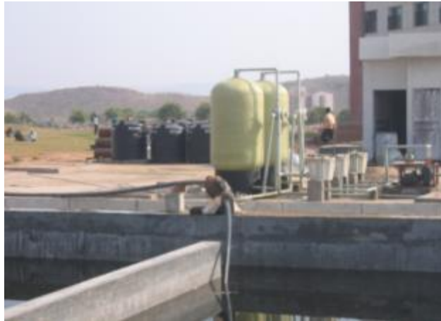
Sewage Treatment Plant
