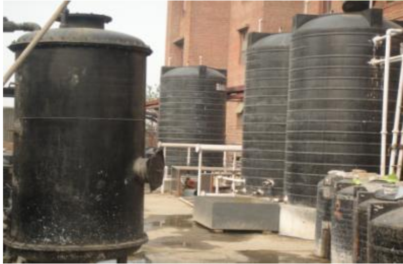
Treated water tanks and Carbon Filter
