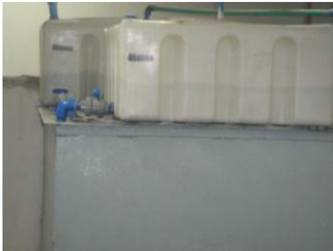
Chemical Reaction Tanks
