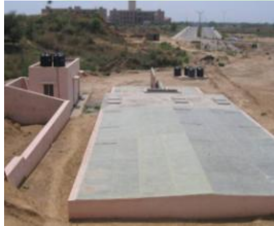
Sewage Treatment Plant 2
